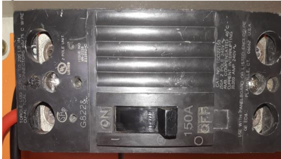
Figura 36. Breaker General Electric
